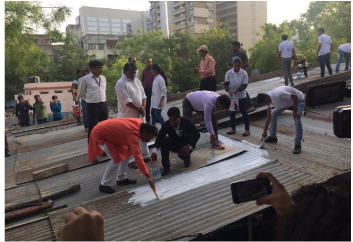
Gautam Shah, Mayor of Ahmedabad, paints the first cool roof in the city (photo: IIPHG-NRDC)
